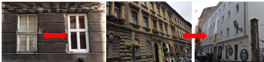
Figure 3: Energetic retrofit with no consideration to heritage value. The original ratios and ornaments are destroyed
