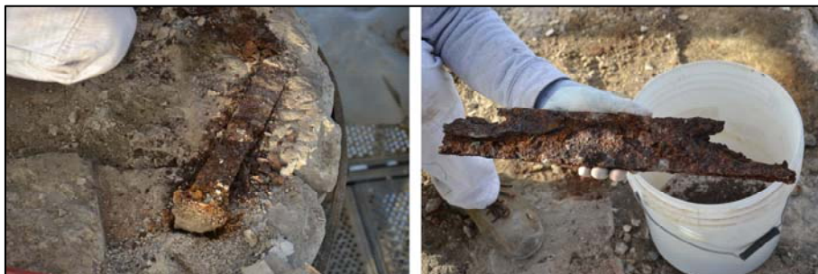
Figure 7: Oxidation of the internal fixtures between the parts which define the individual stone elements of the capital.
