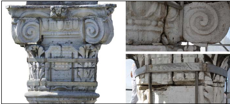
Figure 6: Capital of the column before the restoration works.
