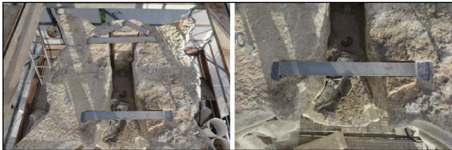
Figure 8: New cramps in duplex stainless steel connecting the various elements of the capital.
